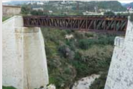
One of the railway bridges built by Australian engineers. The rising sun badge is carved on the abutments
